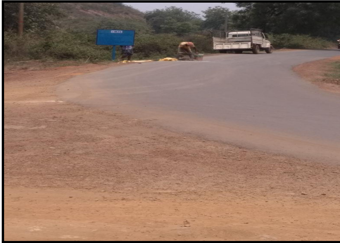
Black topping of road from Radharamanpur village to Jillinda chhak & Arakhapal to Biraramchanderpur Location: Jillinda, Angul District Amount: Rs. 210.13 Lakhs Beneficiary: 20,000 nos. (approx)
